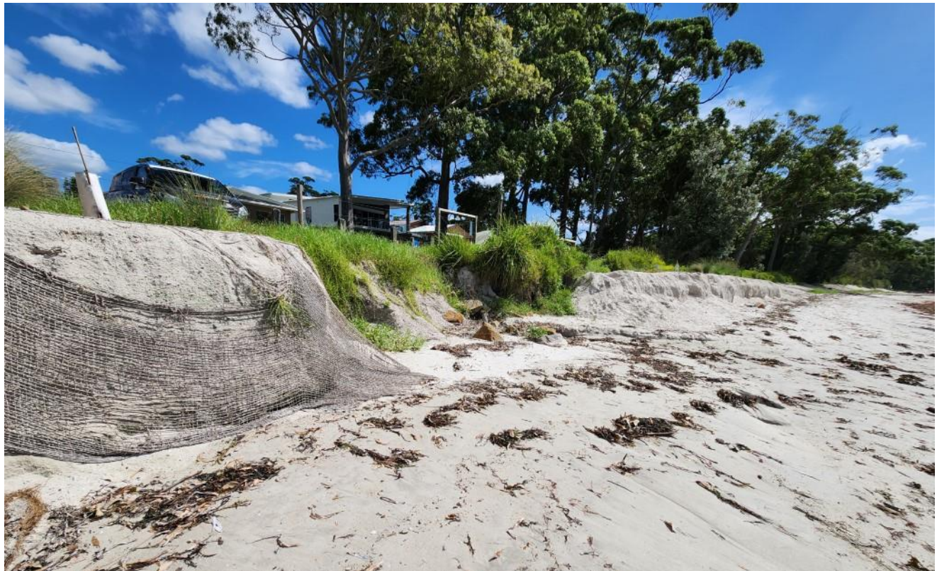
Photo 7. Emergency / maintenance access to beach from Sheaffe St, showing eroded embankment.
